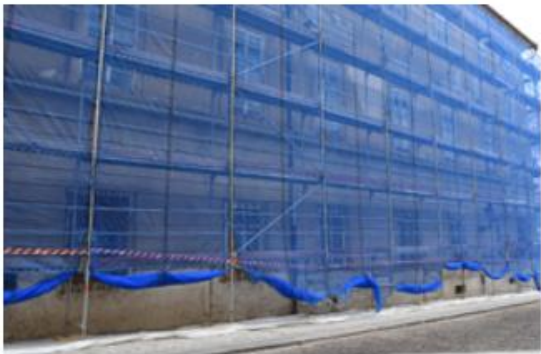
Construction safety nets
